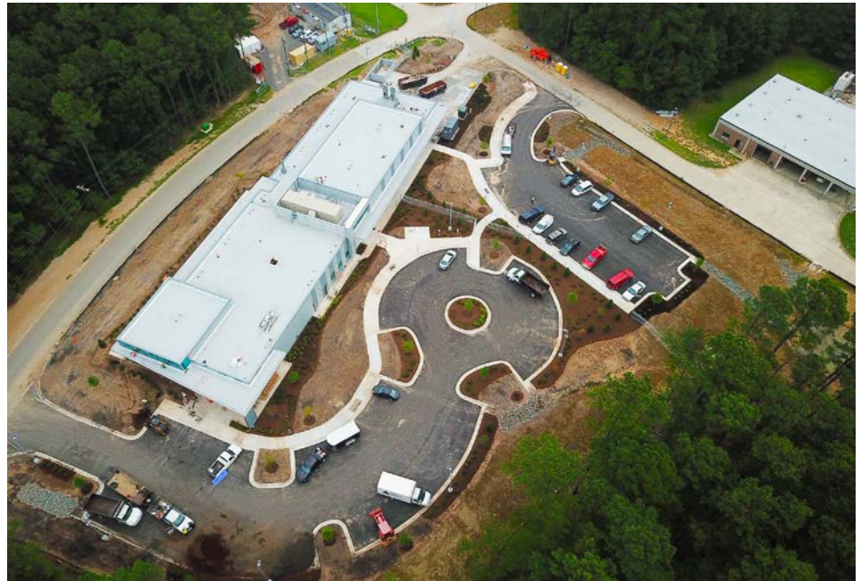
Construction is nearly complete at the Compliance Services building, which houses the state-certified Lab and the IWC/FOG program.
