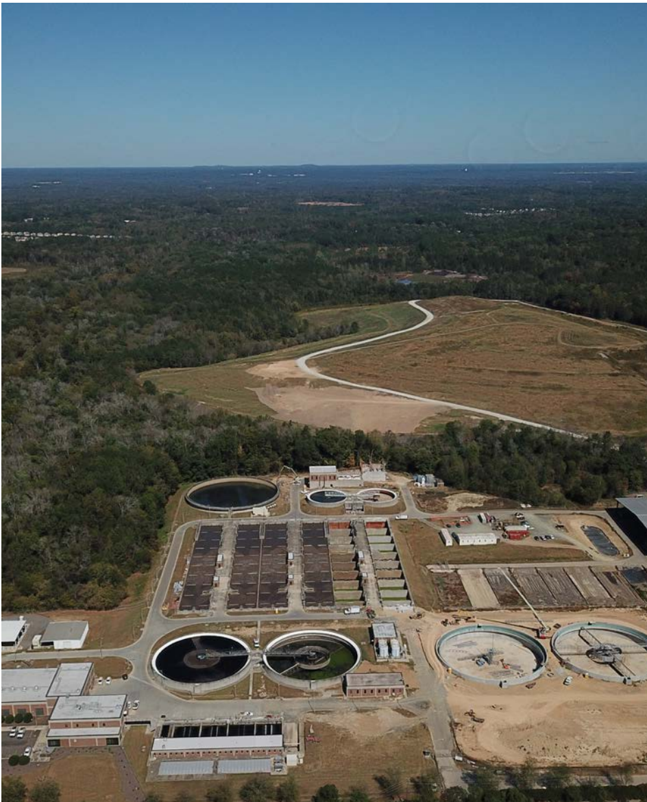
This October aerial photo shows construction on the B side of the North Durham WRF on East Club Boulevard in northern Durham.
